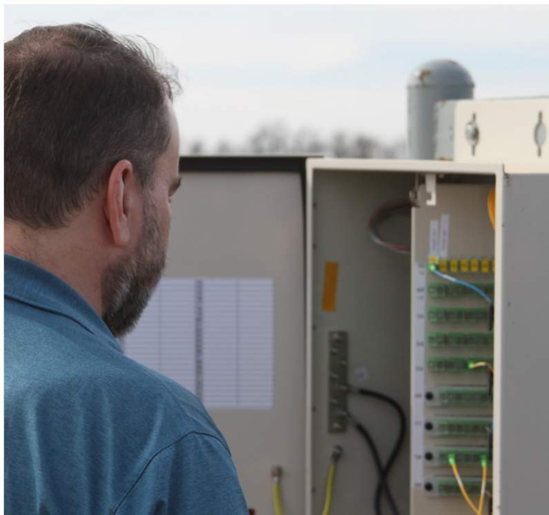
KOBD staff reviews broadband infrastructure during an industry partner site visit for a BAG 2 project in Harper County that was awarded to SC Telcom.
