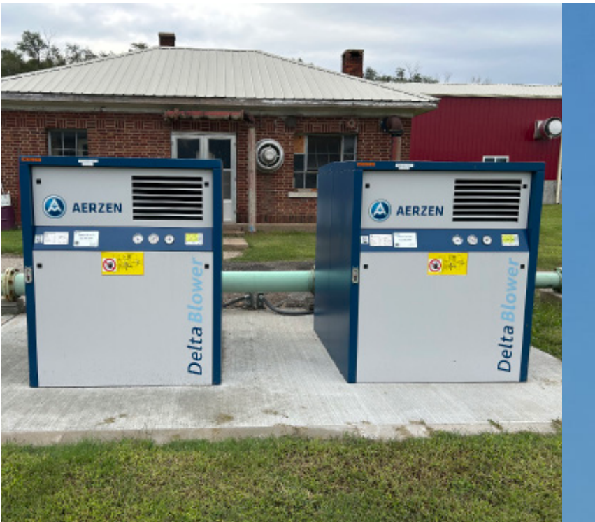
The city of Herington used an Urgent Need grant for the immediate replacement of failed aeration blowers at its wastewater treatment plant.
