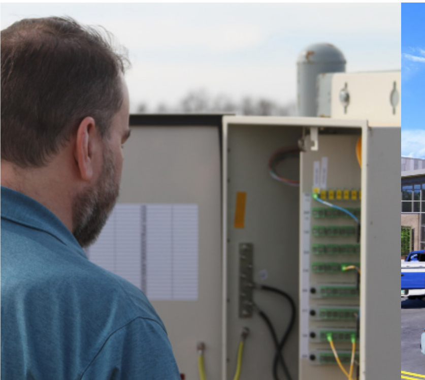
KOBD staff reviews broadband infrastructure during an industry partner site visit for a BAG 2.0 project in Harper County that was awarded to SC Telcom.
